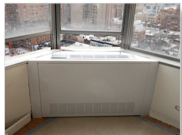
The newly renovated wall housing looks great and the RSK has doubled the capacity from 9,000 to 17,000 BTUs.
