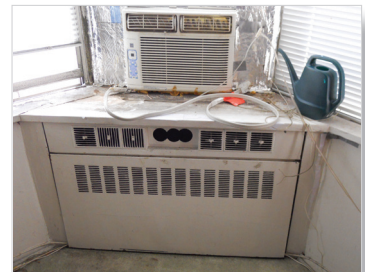
Original units were not adequately cooling these luxury apartments, and many tenants had resorted to adding AC window units, which obstructed their views.
